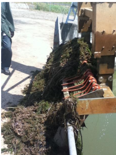
The trash racks in operation catching weed.
