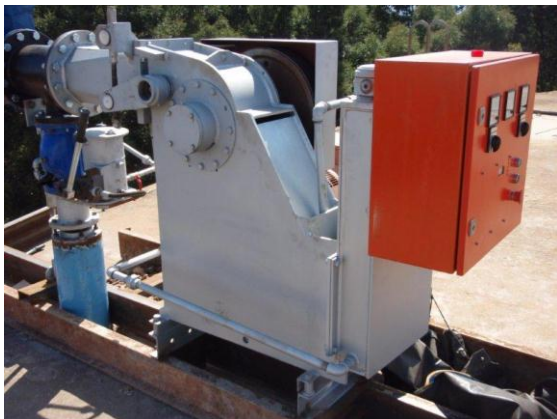
The cross flow turbine at the top of the tank.
