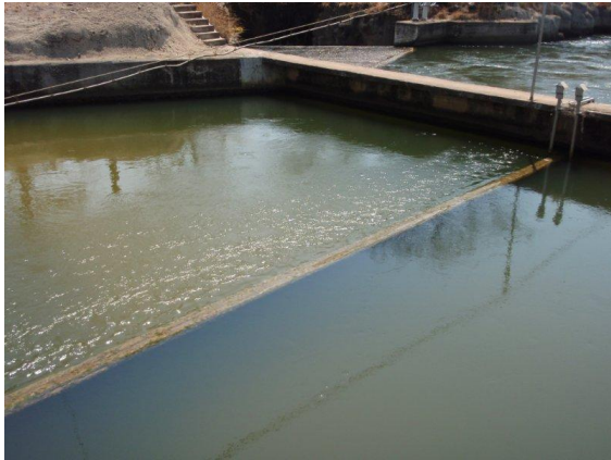
Build-up of silt in the far settling pond.
