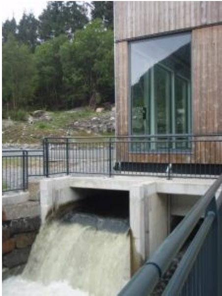
Dalen 1 TailRace, submerged to minimise risk to migrating fish.
