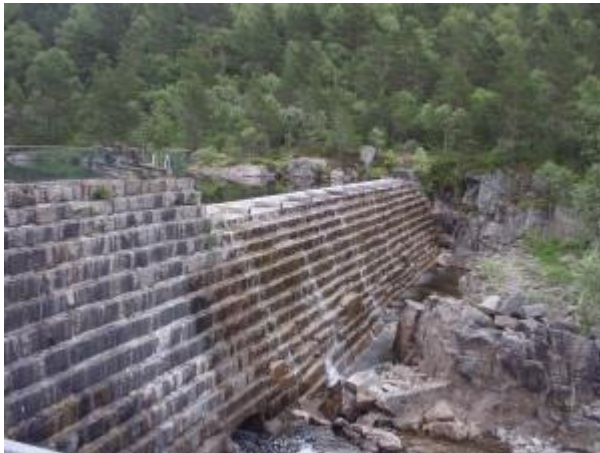
A rather leaky old dam wall.
