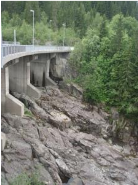
Hydropower dam constructed on top of an existing waterfall on the river Nidelva.
