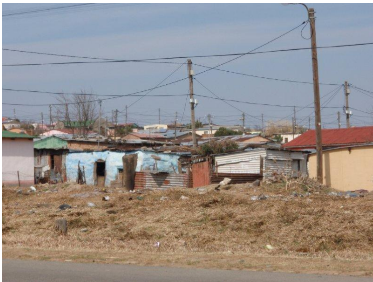
Reticulation of the grid in more built up areas in the Eastern Cape.
