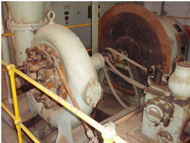
The 1924 turbine and equipment, all still here!
