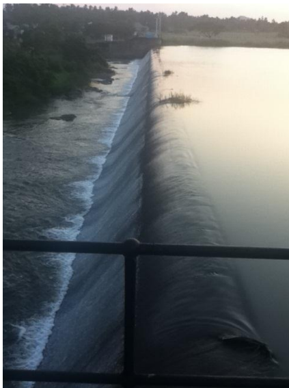
Water spilling from the Hale reservoir, as the site is shut for rehabilitation.
