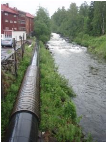
A section of wooden pipeline in the penstock to Andreas' powerhouse.
