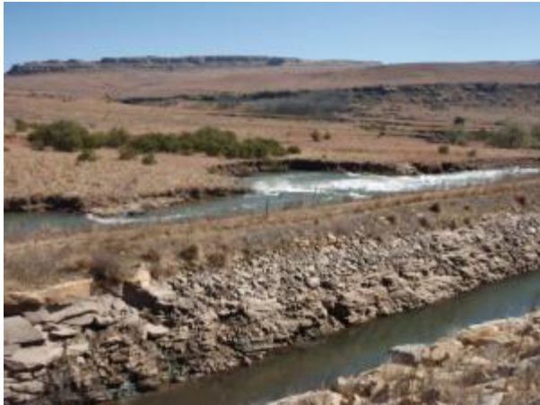
Inlet canal adjacent to Ash river; note washout in the river.
