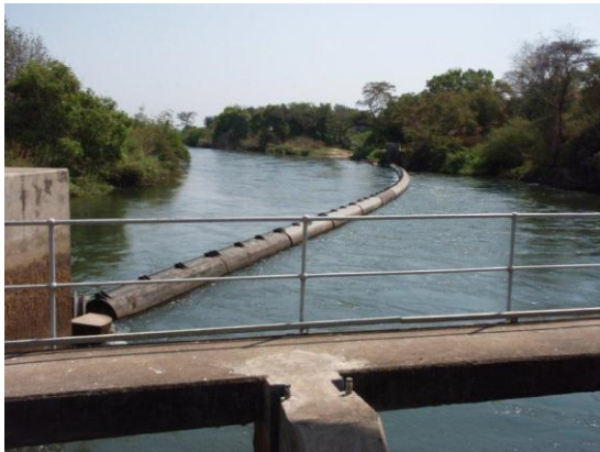
Boom in front of intake to prevent hyacinth entering intake.
