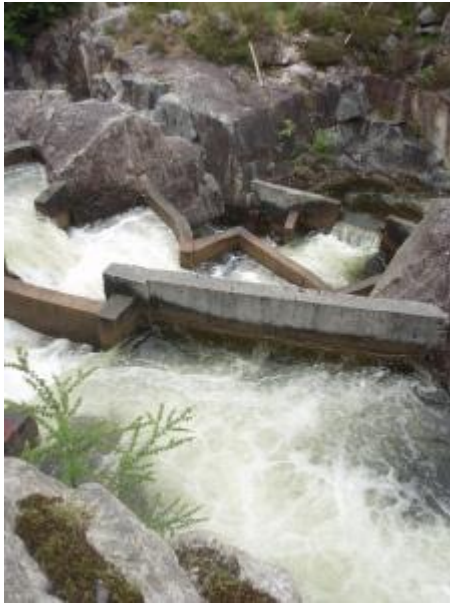
The fish ladder that doesn't work!
