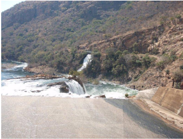
Looking down from the dam wall; note the flow on far side, coming from turbine house.
