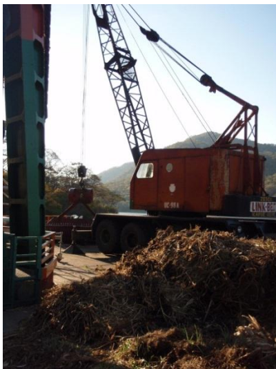
The crane on an endless cycle of lifting hyacinth weed out of the intake area.
