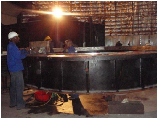
Workers underground in the plant working on the runner for Turbine 4, as part of the rehabilitation project.
