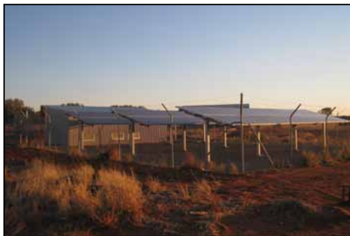
Bushlight solar array at Ulpanyali
