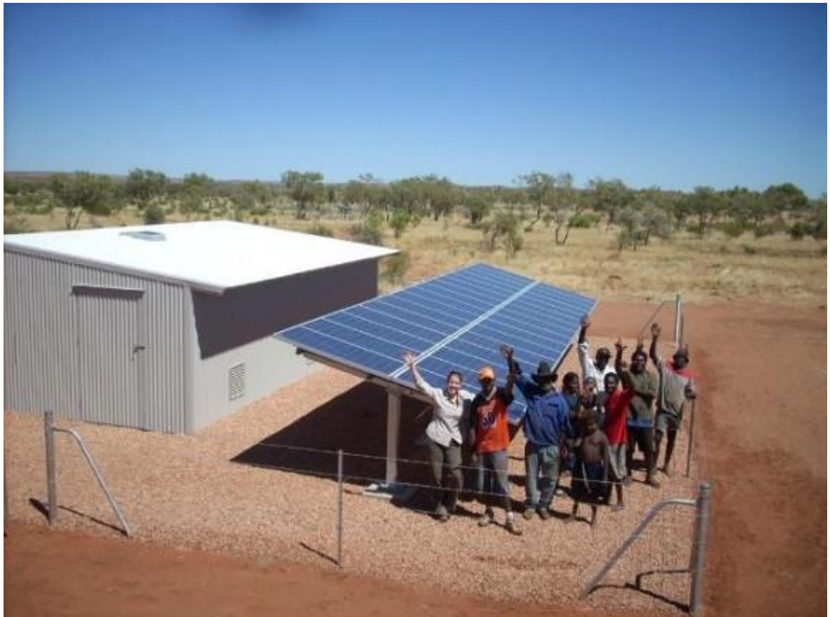
Community RE System showing PV array and shed housing battery and generator
